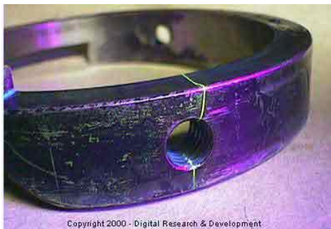
Magnetic particle wet fluorescent indication of a cracks at a fastener hole
