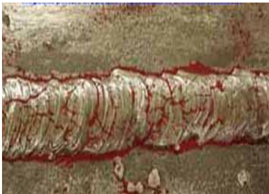
Indication of cracks in a weldment
